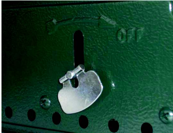
Figure 8 Auxiliary Burner Control
